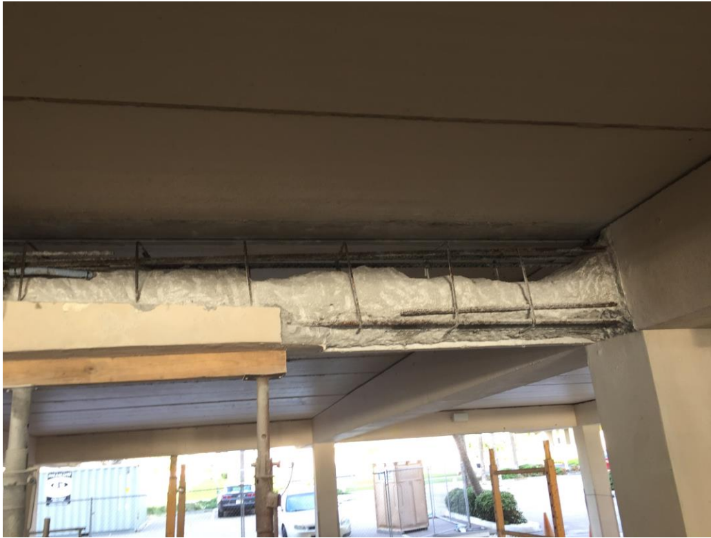
Picture 1: Beam that will be fully replaced
