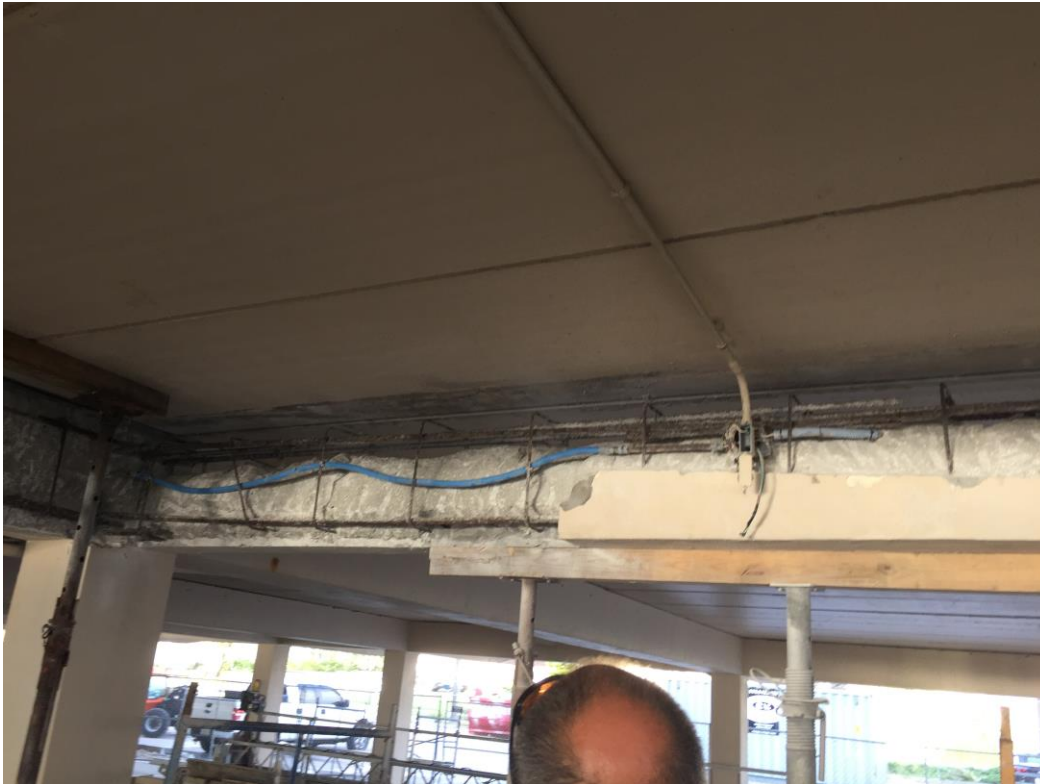
Picture 2: Beam that will be fully replaced
